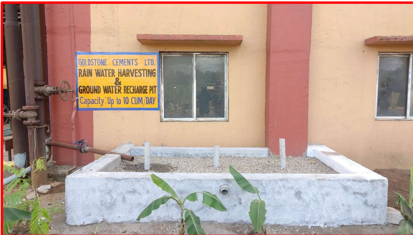
Rooftop rainwater collection and ground recharge system at CPP
