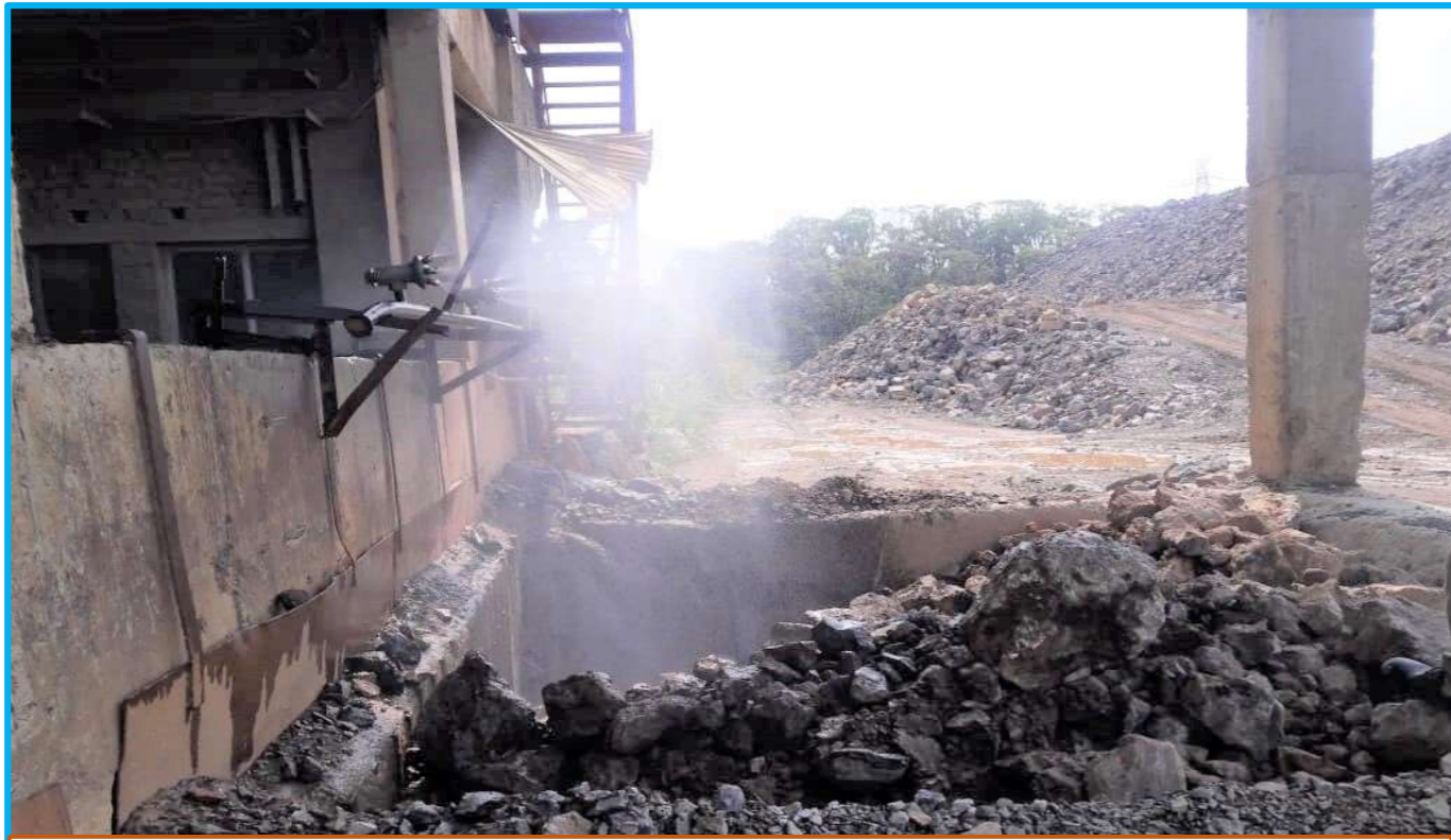
Water Sprinkling through Permanent Water Sprinklers at Limestone Crusher
