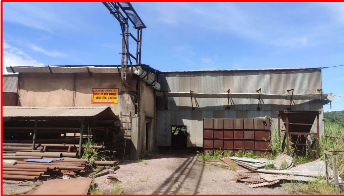
Rooftop rainwater collection and harvesting system at CPP water reservoir
