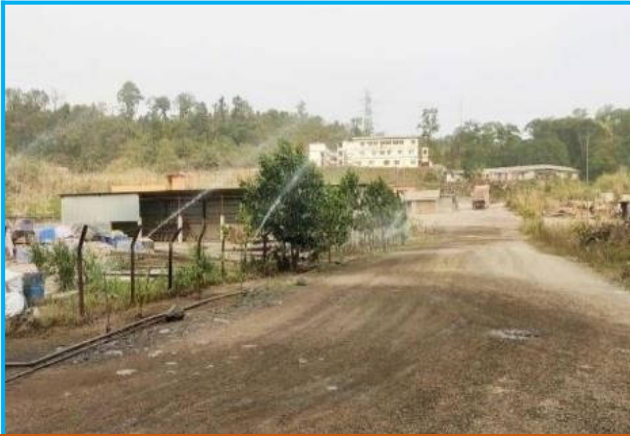
Water Sprinkling in roads through Permanent Sprinklers in material yard surrounding roads
