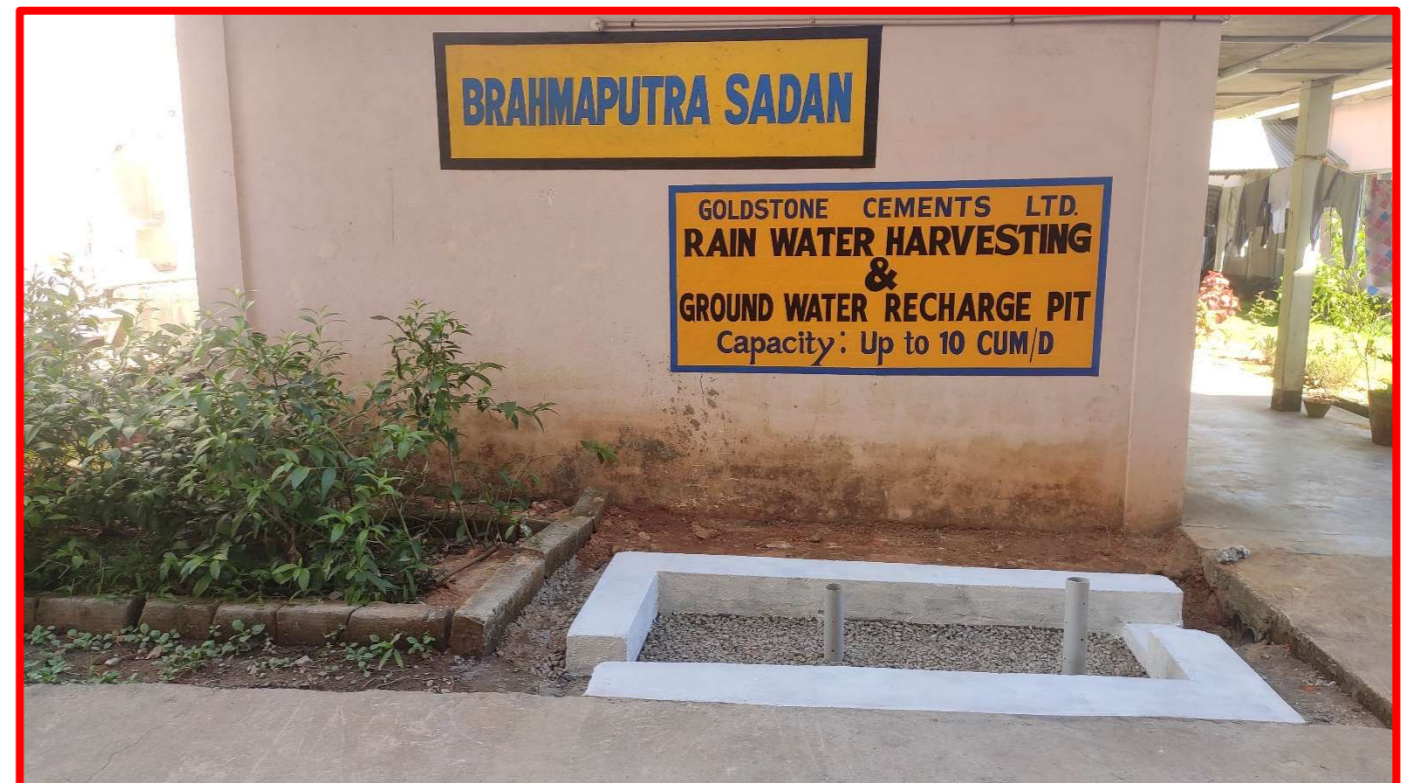
Rainwater collection and ground recharge system at Guest House (Brahmaputra Sadan)
