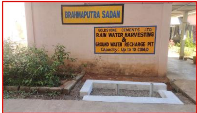
Rainwater collection and ground recharge system at Guest House (Brahmaputra Sadan)
